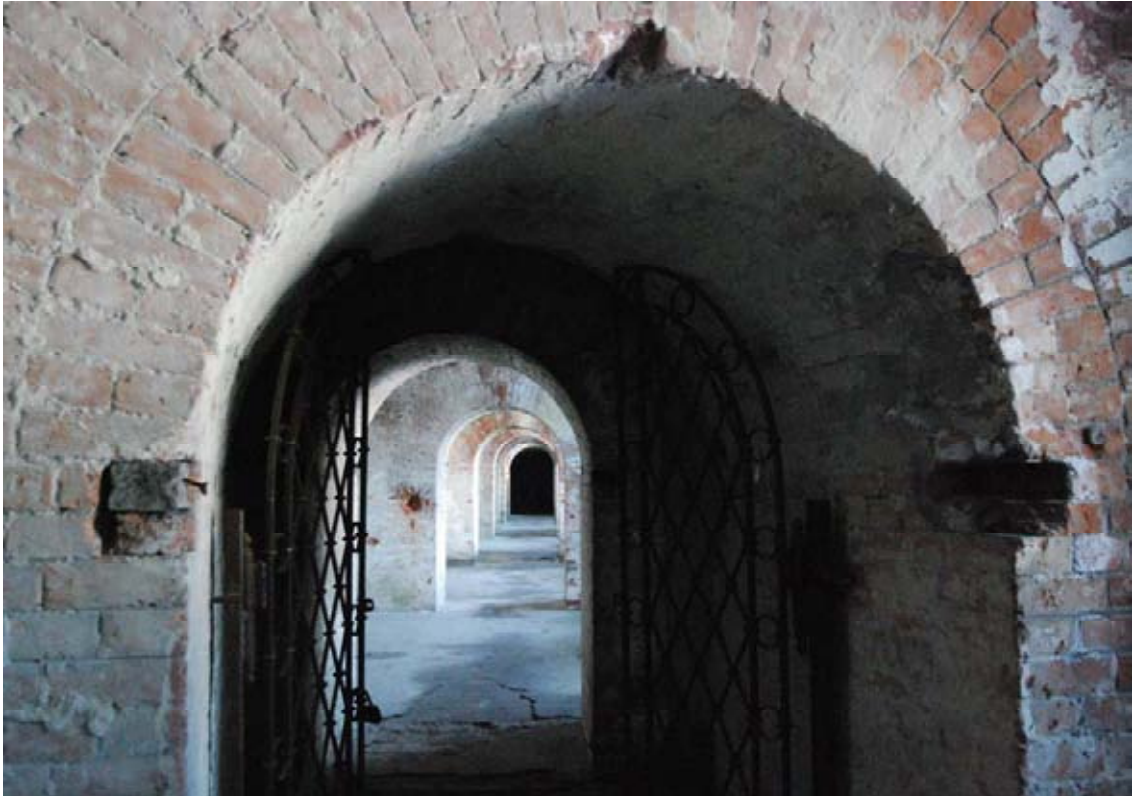
Impression in Fort V. Conservation of cultural heritage, combined with natural values. In the crack left from the gate a serotine has its hibernation place.
